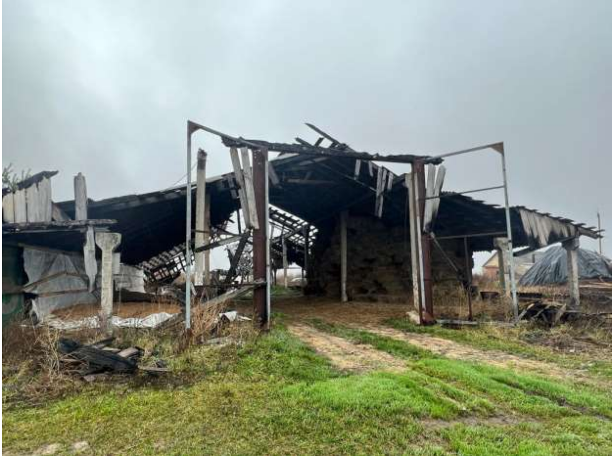
Destroyed production buildings of the "Svitanok" family farm. The village Pochepin, Bucha district, Kyiv region. 16 November 2022. Photo credit: The Institute of Economics and Forecasting of the National Academy of Sciences of Ukraine
